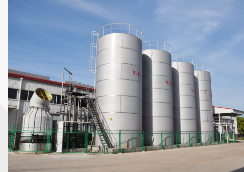
Raw Material Tank Area
