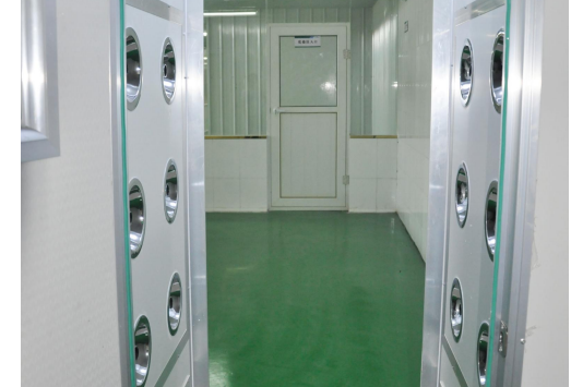
Air Shower Room
